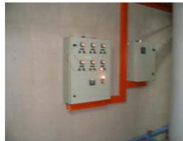
Backup Heater panel
