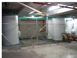
Hot water Storage Cylinders
